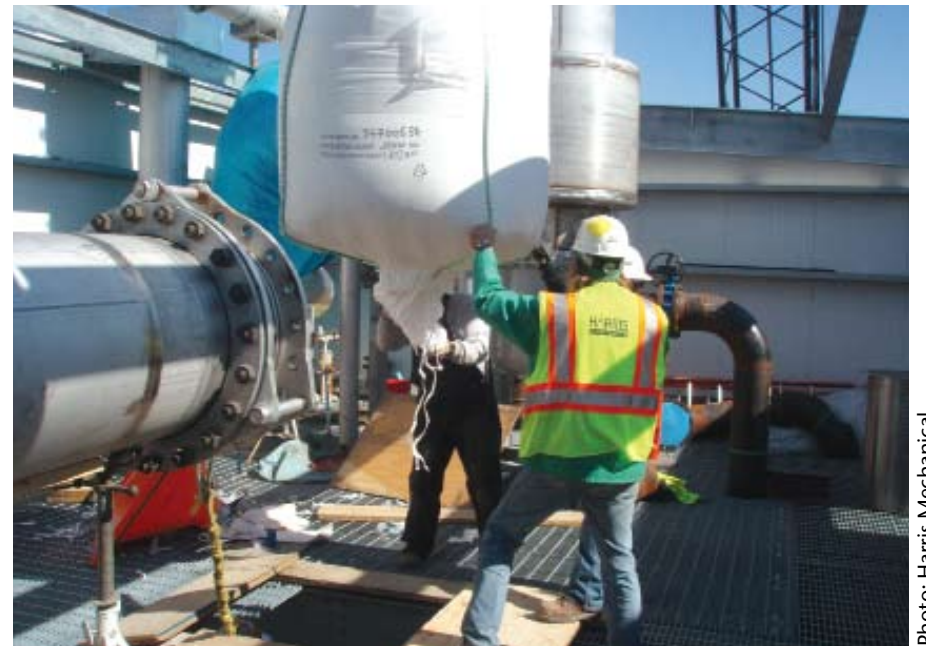
Photo: Harris Mechanical
