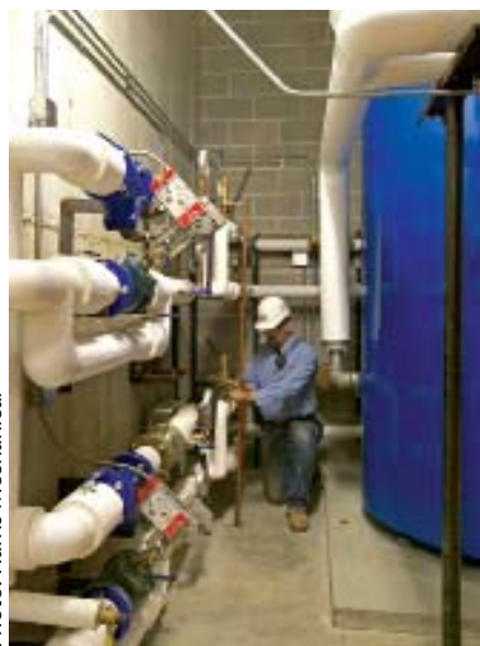
Photo: Harris Mechanical
