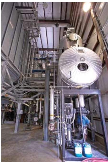
Below, a mechanical room installed by Berg.
