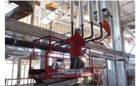
A technician with St. Cloud uses a JLG lift to inspect ductwork.
